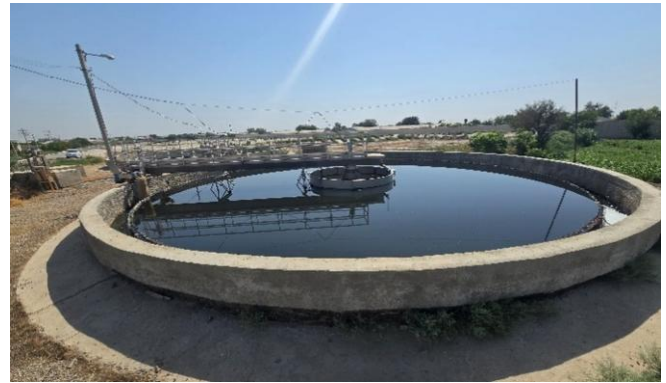
Wastewater treatment facility used for three-stage treatment
