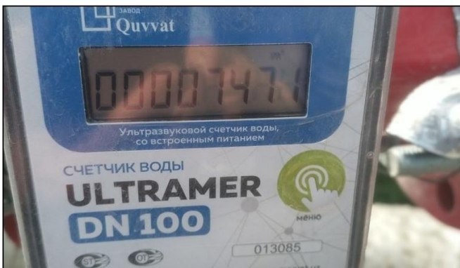
Metered water monitoring
